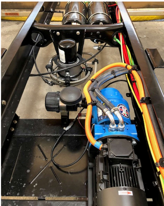
Air Comp & Air Dryer
