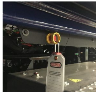
A lock properly installed on an eCascadia's emergency stop switch.
